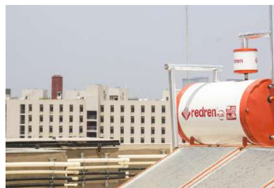
b) Housing solar water heaters
