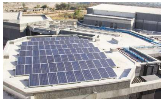
a) Academic building PV panels
